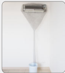
One drainage pipe
